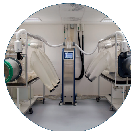
ScanClime supplying humidified/dehumidified air to isolators
